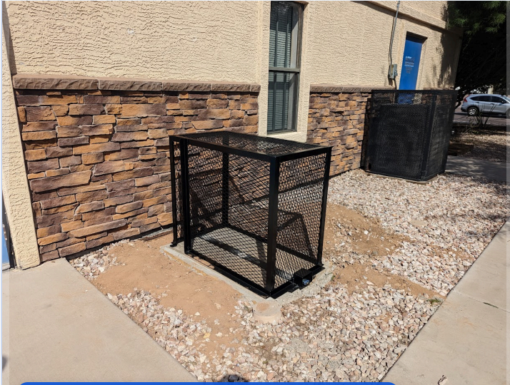
CUSTOM HVAC EQUIPMENT SECURITY CAGES
